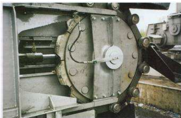
The self-adjusting chain sprocket mounted on the portal reclaimer
